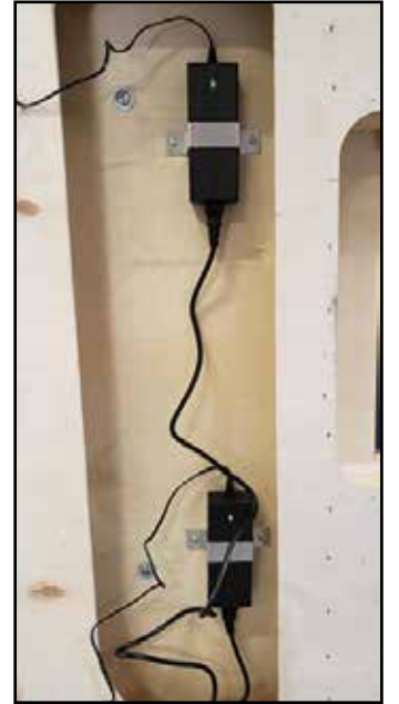
Transformers on back of panel
